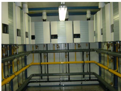
CV ketels in container
